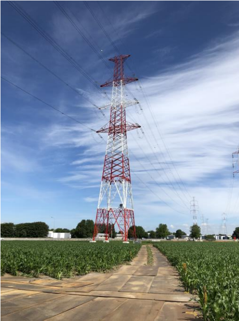
Figuur 26: Rood-wit bebakende mast
